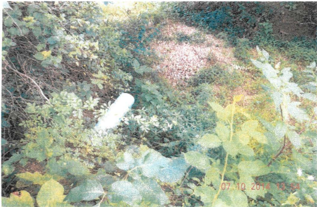
DSCN2162, Spot erosion in the bottom of the tributary directly beneath the pipe
